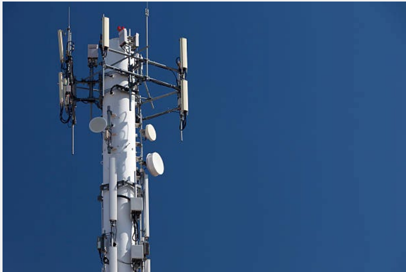
Base station tower
